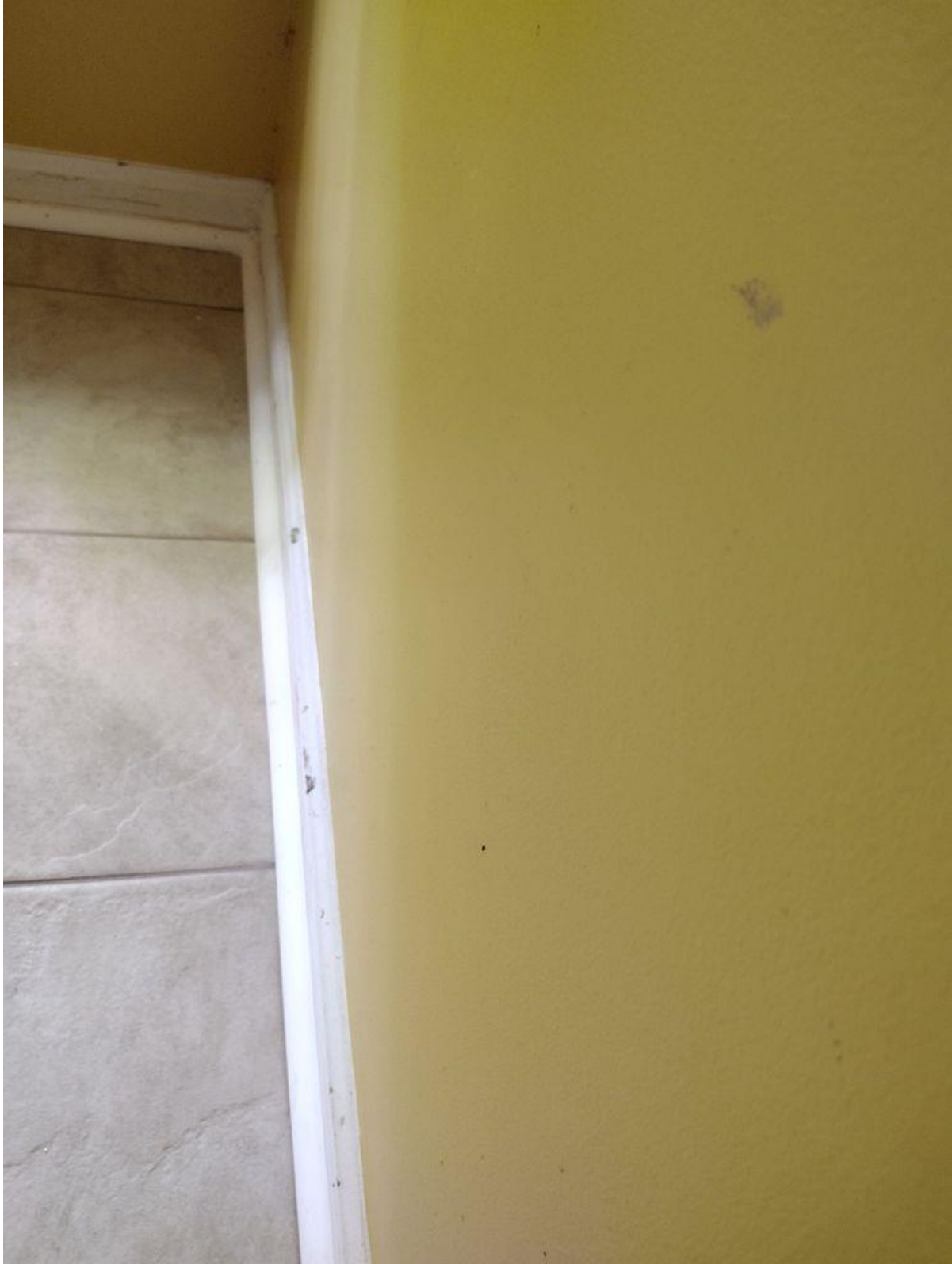
Grout on walls, Photo 6. Grout and thinset smeared on walls and baseboards.
