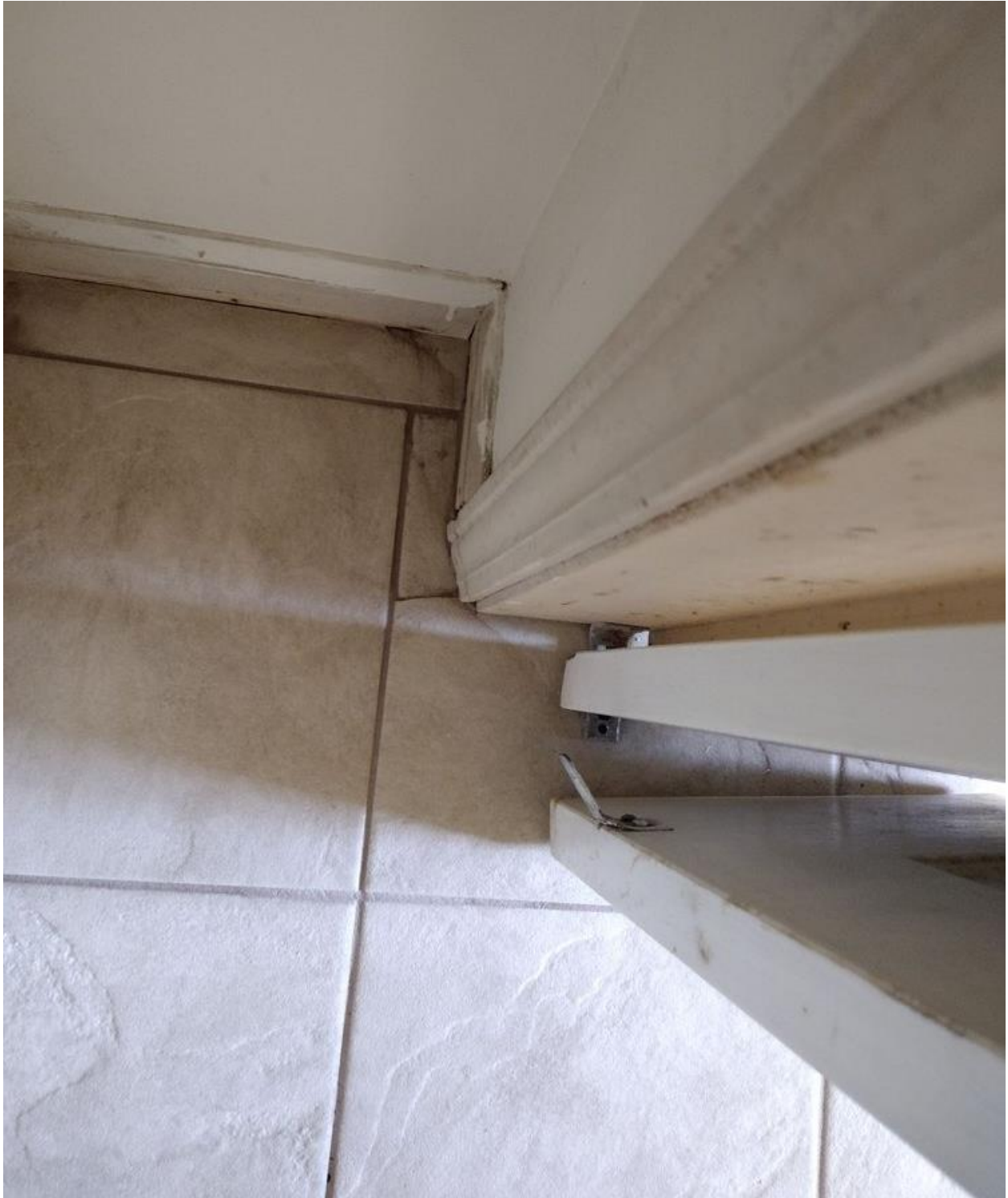
Tiles installed broken, Photo 1.
