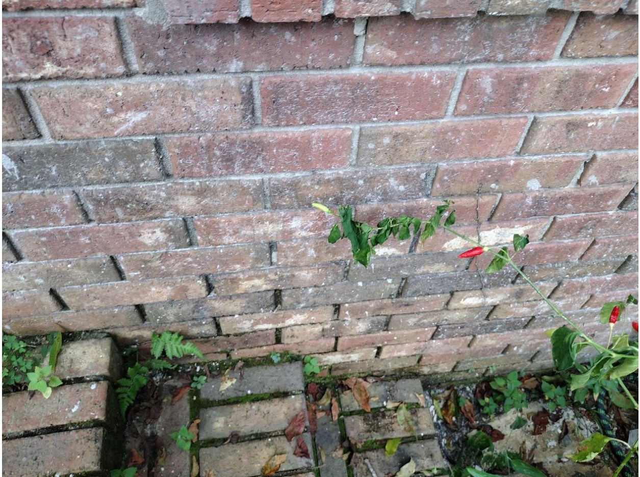
Thinset on brick porch, Photo 7. Thinset splattered onto brick siding.
