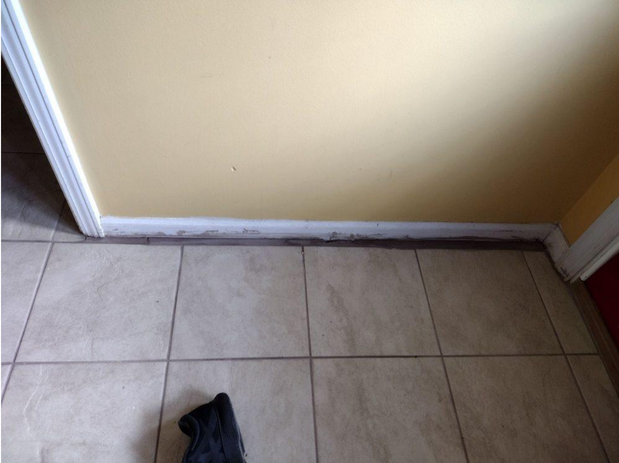
Grout on walls, Photo 5.
