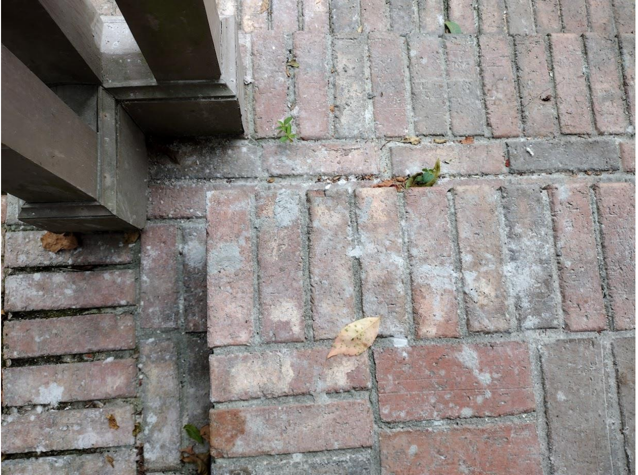
Thinset on brick porch, Photo 11.
