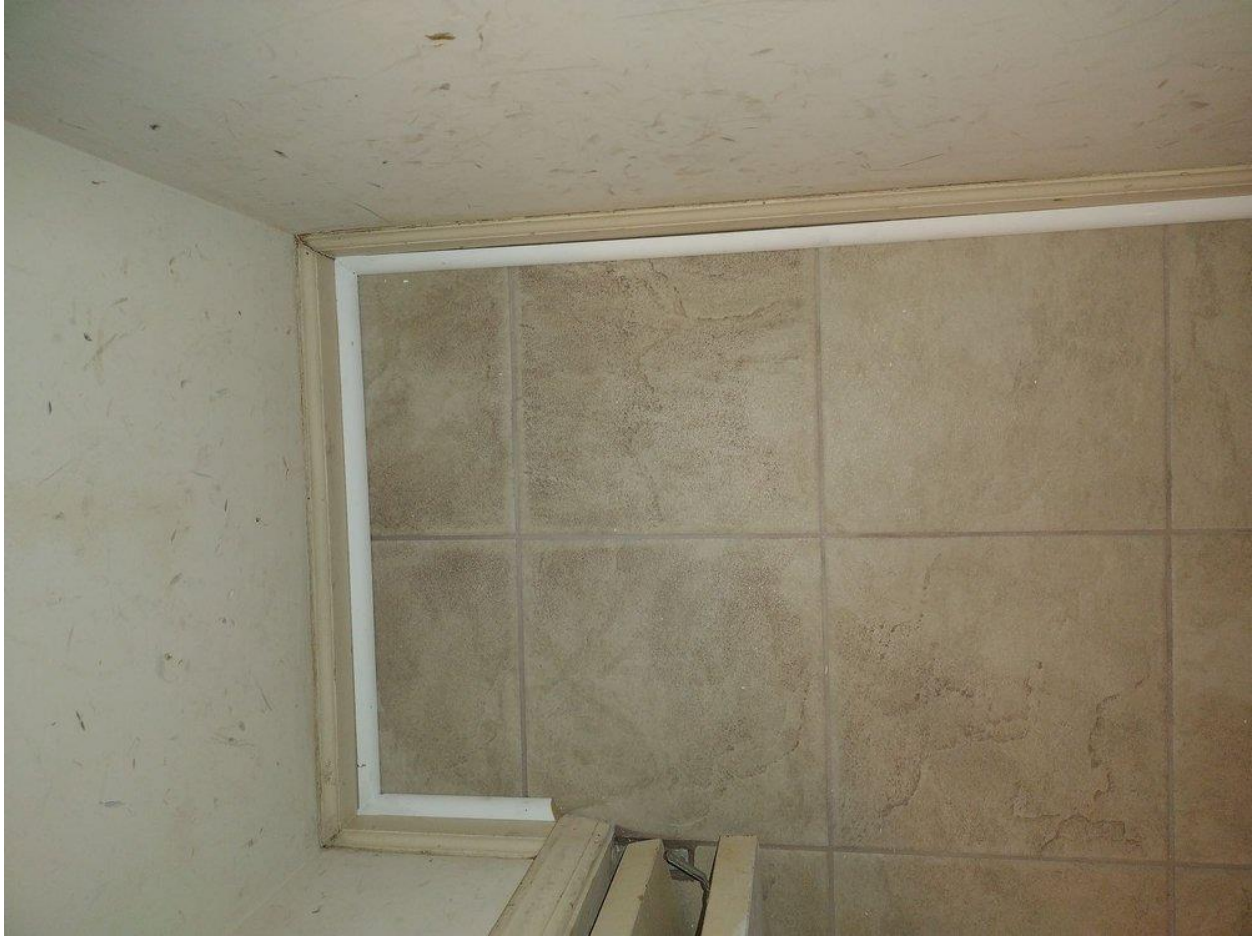
Grout cured on top of tiles, Photo 4. Grout smeared on top of tiles for a permanently dirty look.
