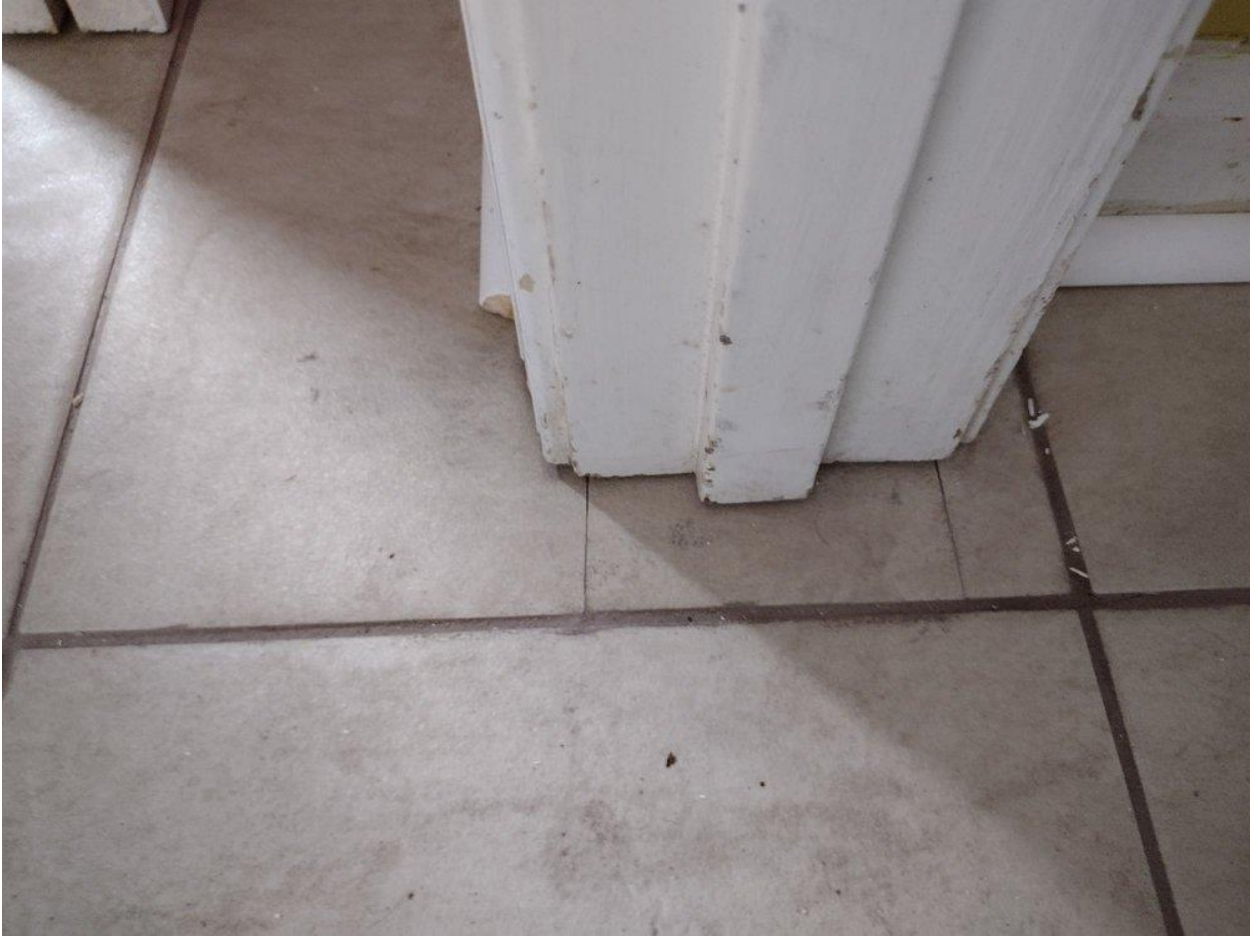
Tiles installed broken, Photo 2.
