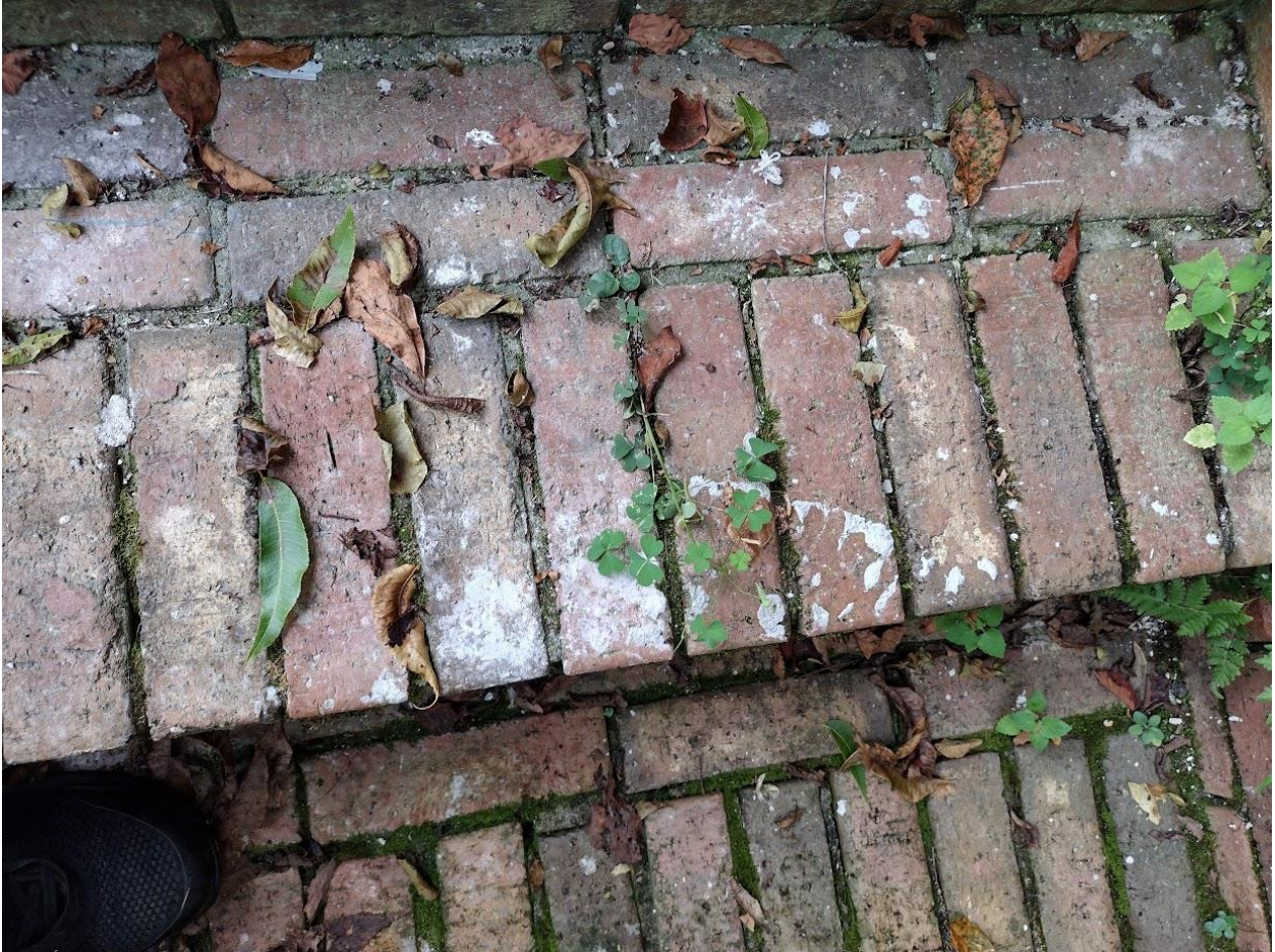
Thinset on brick porch, Photo 9.
