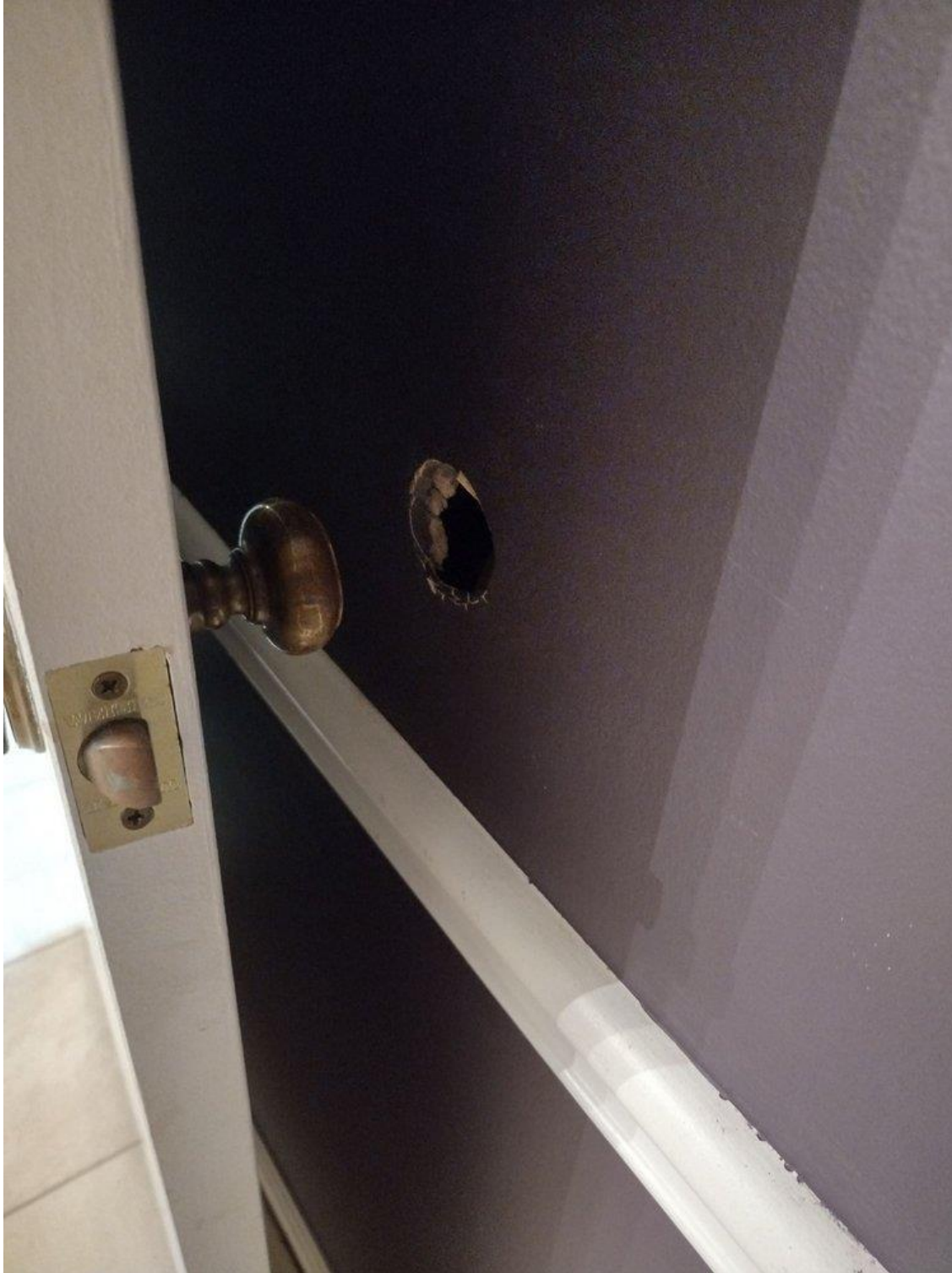
Wall hole, Photo 1.
