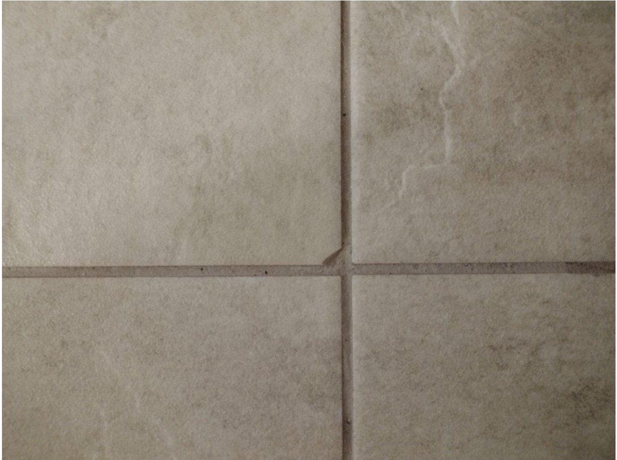
Tile installed chipped, Photo 1.
